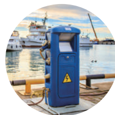
Habor Electrical Outlets
